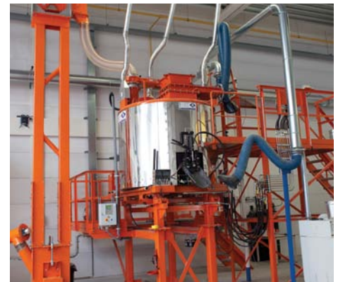
Mixing equipment installed at Shell Thiocrete prototyping facility, near Amsterdam.
