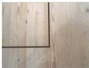
Sharp-edged corners on NVI/IVI panels
