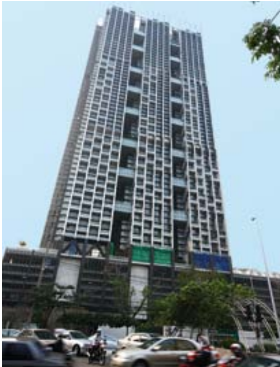
MET, Bangkok, Thailand High class residential building with 3 KONE JumpLifts and 2 Construction Time Use (CTU) elevators.
